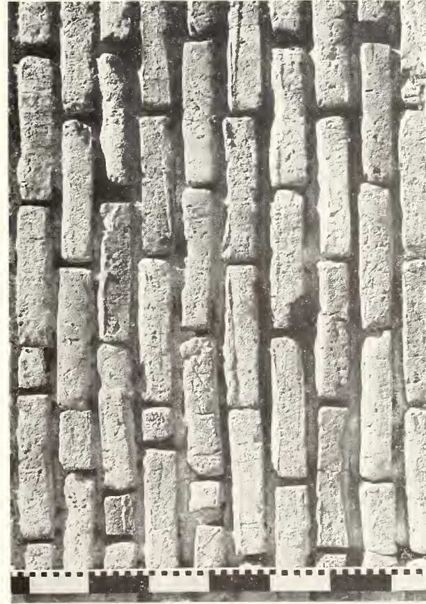
PHOTO. M. B. SMITH, NEG. L-93.23 FIG. 42—SANCTUARY, EXTERIOR, BRICKWORK AT NORTH CORNER
